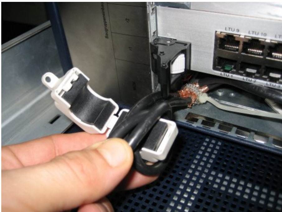
Figure 44: Looping the DC cables through the ferrite core
