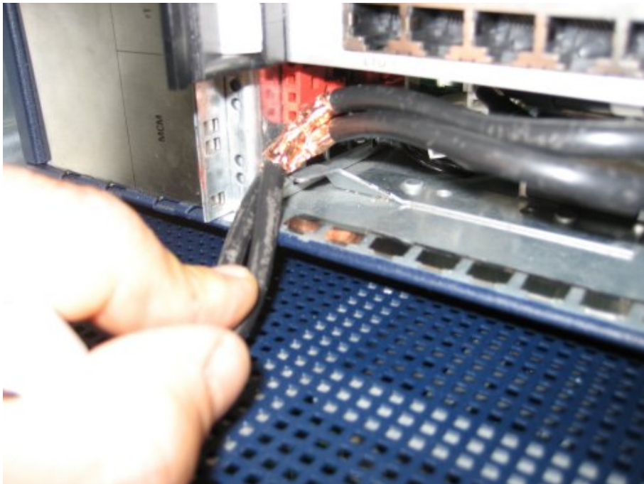
Figure 40: Stripped DC cable
