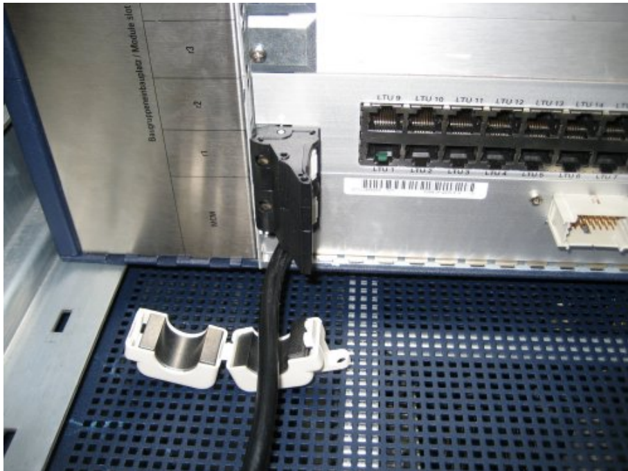
Figure 37: Opened ferrite core below AC cable
