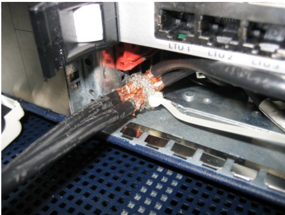
Figure 44: DC cable shield on housing
